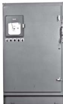
300 HP 600V Starter in Type 3 Enclosure
