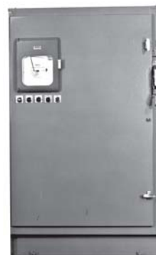
400 HP 600V Starter in Type 3 Enclosure
